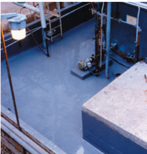
Stonhard's Stonchem 677 lining provides an effective secondary containment system for this sulfuric acid containment area.
