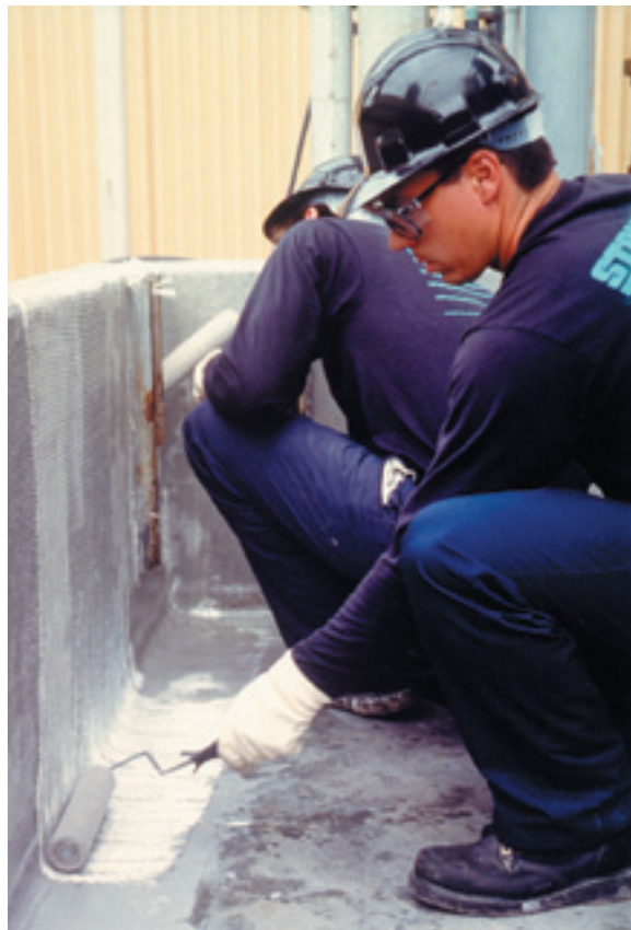
Stonhard installation teams provide trained attention to details and superior preparation to ensure a high-quality installation.
